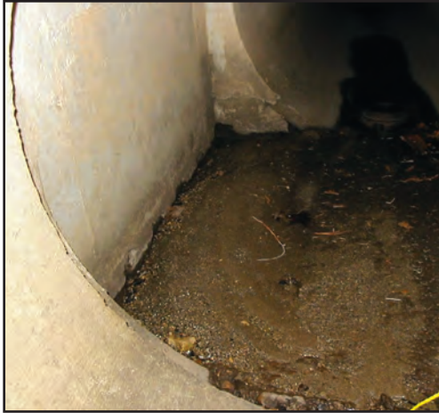
Figure 20. Accumulation of sediment in the junction of a manhole with the storm-sewer conveyance system.
